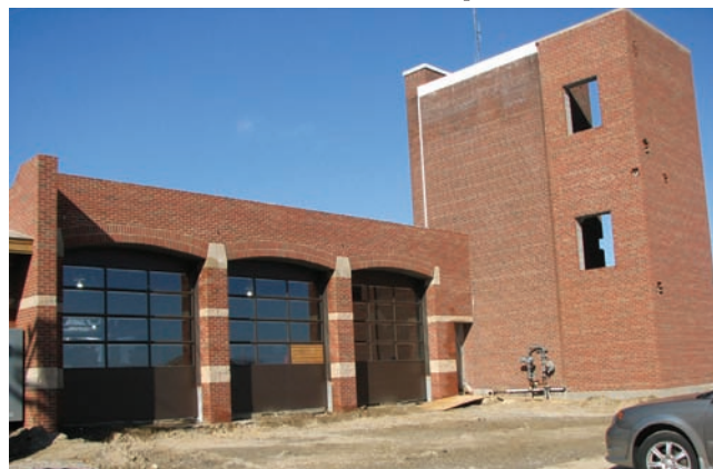
Construction of the Central Fire Station will be completed and equipment moved in July 2009
