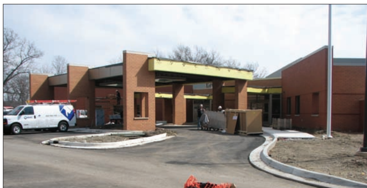
The new Senior Center, part of the Township’s Capital Improvement Program, is nearing completion
