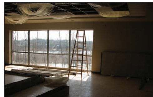
Finish work is being done on the interior of the Senior Center.
