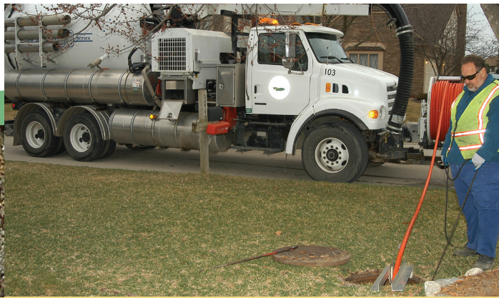
FOG build-up in sewer pipes (shown below) is costly to clean requiring local public works staff to go to the site and remove the blockage (shown above).
